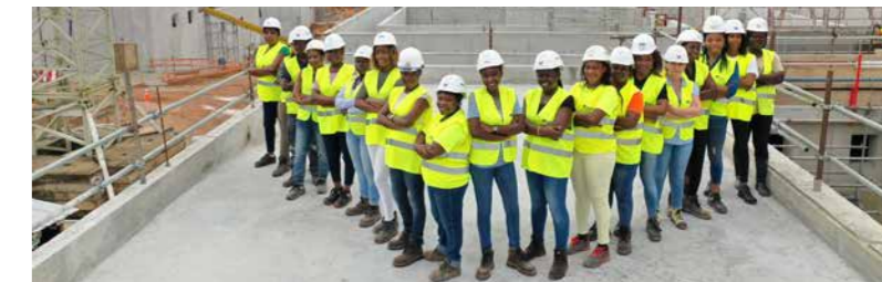
Civil engineering works of Water treatment plant, La Mé, Ivory Coast One of the biggest WTP in West Africa: treatment and distribution of 240,000 m 3 of drinking water every day (around 30% of daily water consumption of Abidjan in 2025).
